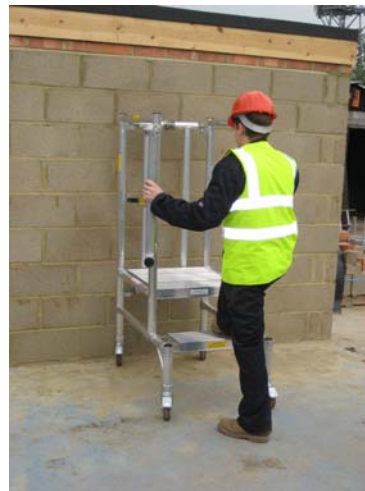
6 ) USE STEP TO ACCESS PLATFORM
