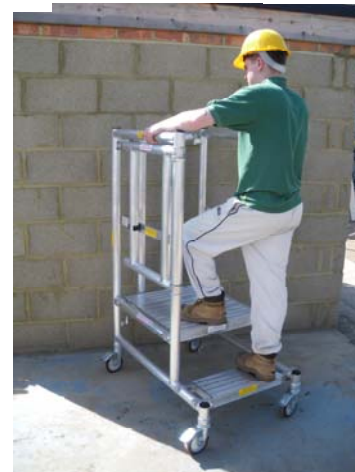
RELEASE GATE, SWING ROUND AND LOCK BEHIND YOU ON THE VERTICAL BEFORE USE.
